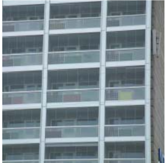
PV in balcony parapets.
