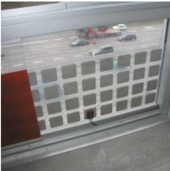
Sliding screen and PV installation.
