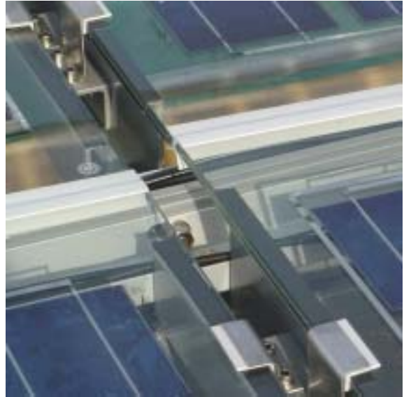
Detail of PV installation.
