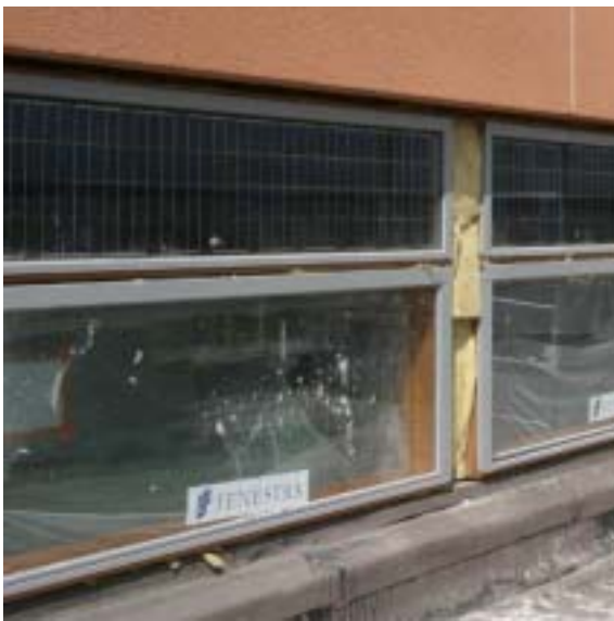
Window integrated PV installation.
