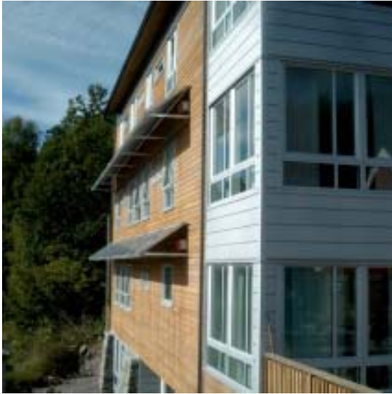
PV solar shading devices at the facade.
