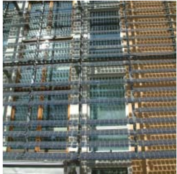
PV installation on metal frame in front of facade.
