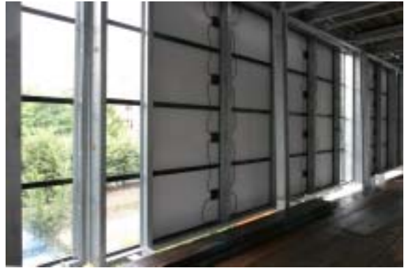
PV panel back.
