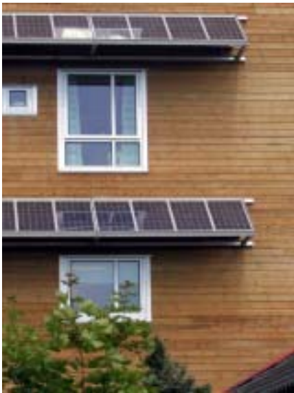
PV panels above the windows.
