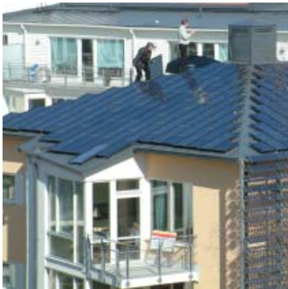
Roof top PV installation.
