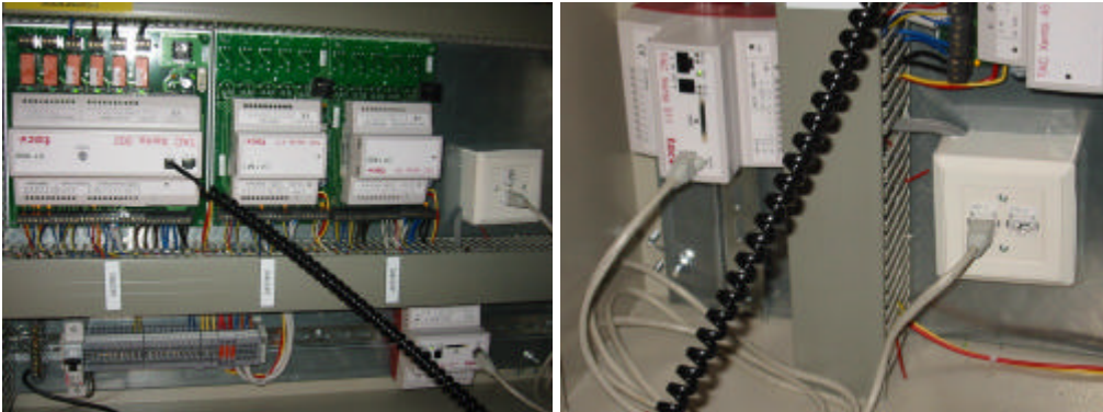
Figure: I/NET LAN ICT approach for building automation and remote monitoring through internet at Skanska/Ekoviikki in Helsinki (source SOLPROS 2002).
