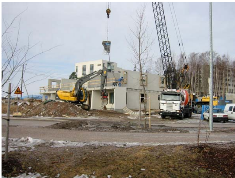
The YIT building under construction in Ekoviikki, February 2002 (photo SOLPROS). By the end of 2002, the building will be equipped with innovative PV-balcony modules.
