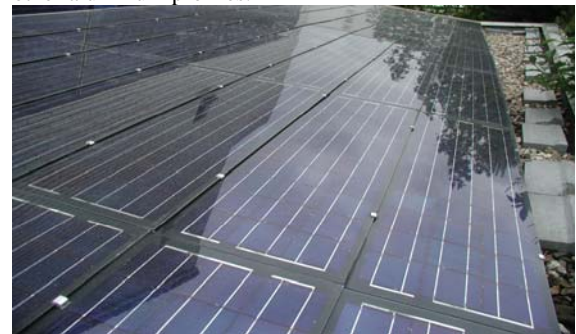
Photo 3: SolTile2 PV roof integration without modules frames or aluminum profiles (Utrecht-1, Netherlands)
