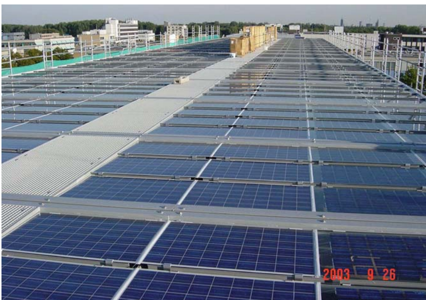
PV Pergola mounted and ready for use.
