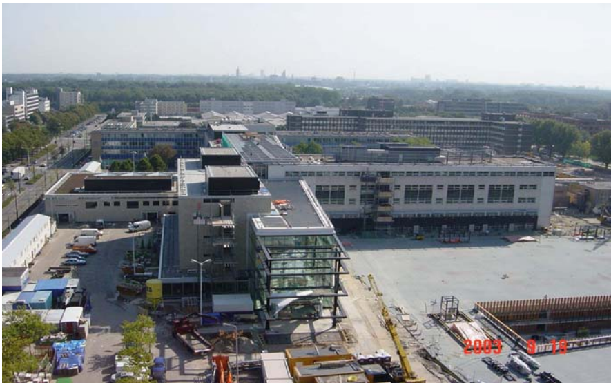
Overview (PV Pergola in the middle)
